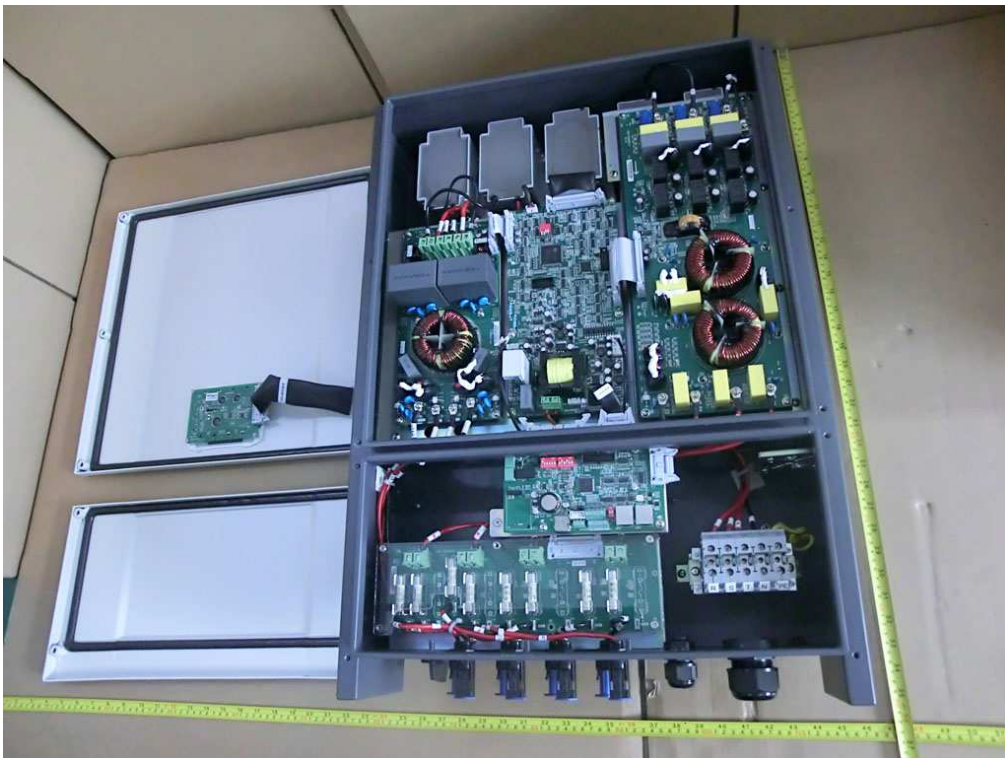
Internal view of the unit
